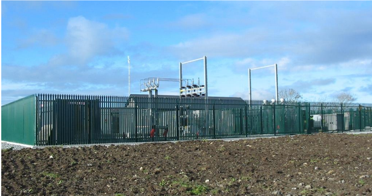
Figure 2-12 Typical Substation Compound
